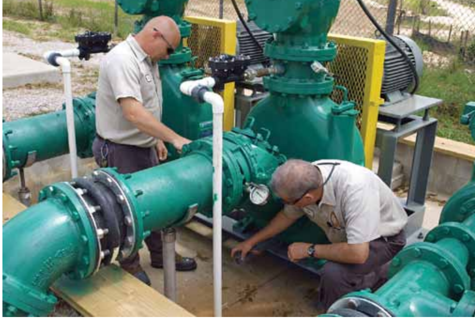
Lee Gilley (left) and Dan Davis perform planned maintenance on the plant's Gorman-Rupp suction lift pumps.
