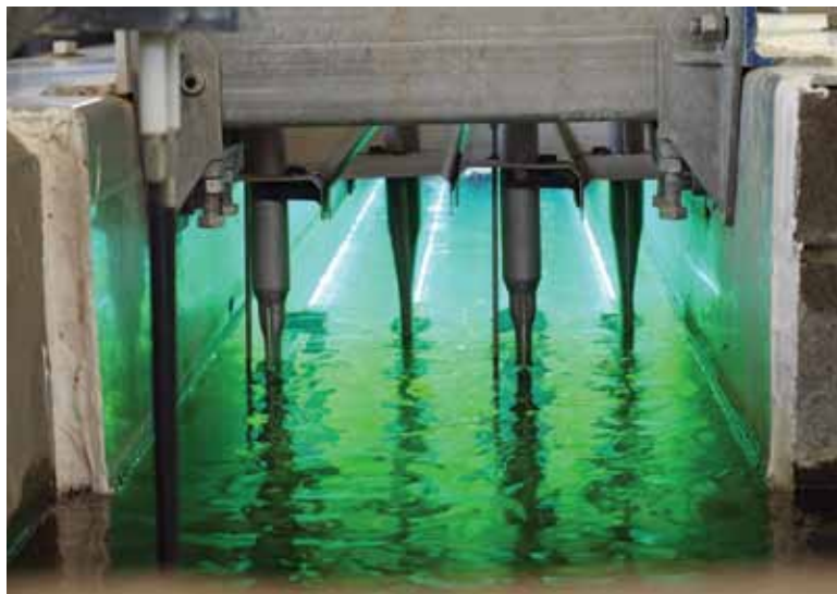
UV lights on the facility's Trojan disinfection units.
